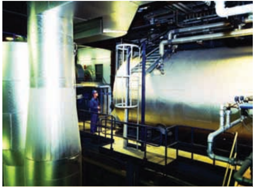
Left: the Energos plant in Stavanger, above: inside the energy from waste plant
